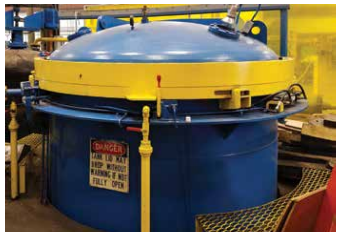
8-ft. Vacuum Pressure Impregnation (VPI) System at EECO's Industrial Motor Services in Richmond, VA
