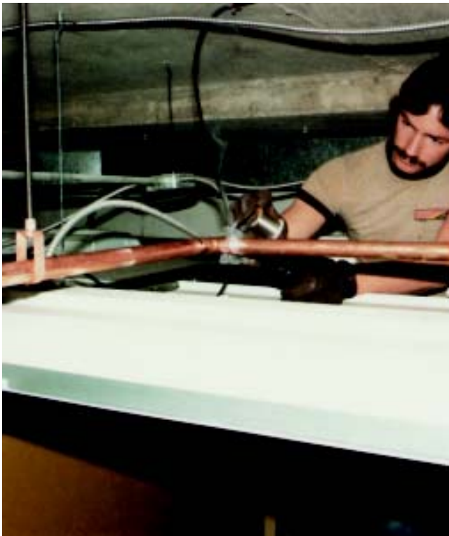
Figure 1. Copper fire sprinkler system in a commercial building being installed with electric resistance heating.
