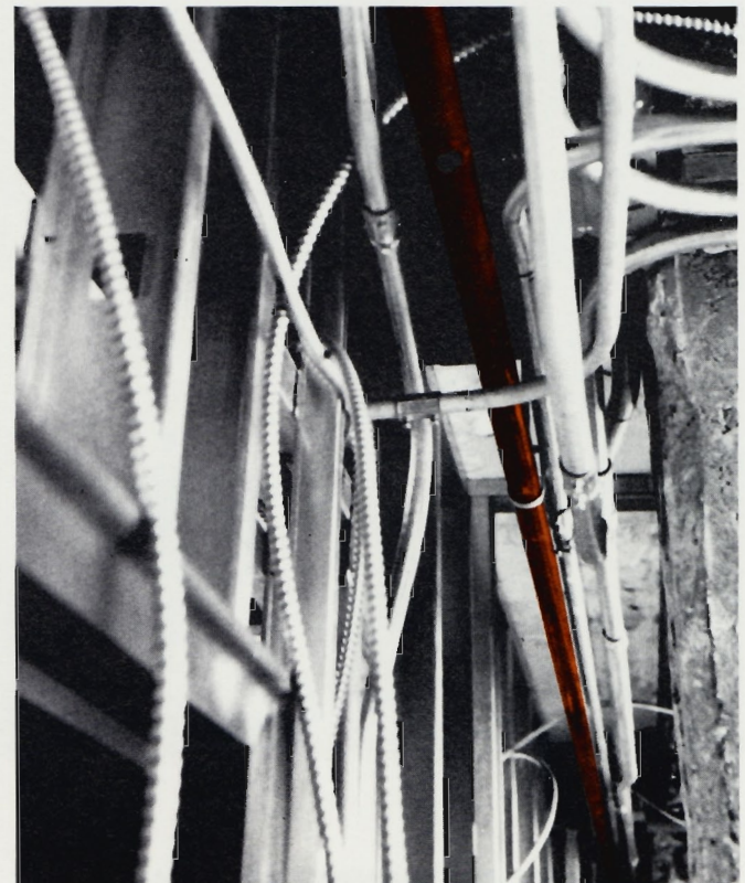
Figure 5: Tube run with field installed T-connection.
