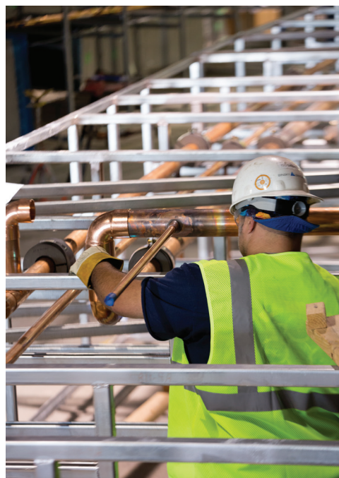
A plumber prepares the copper piping on racks at the warehouse. Photo Credit: Angela Richardson Photography
