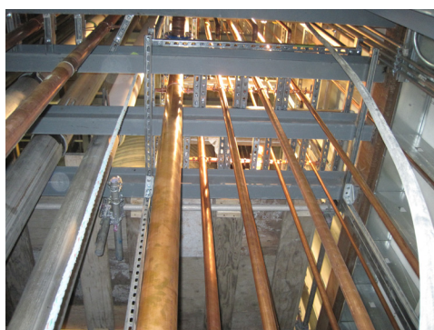
Copper tubing used for a medical gas installation at a hospital. Photo credit: CCBDA
