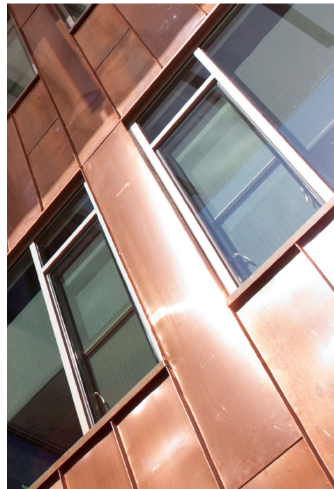
Exterior copper wall panels, Willamette University. Photographs by Michael Mathers courtesy of Henneberry Eddy Architects, Inc.
