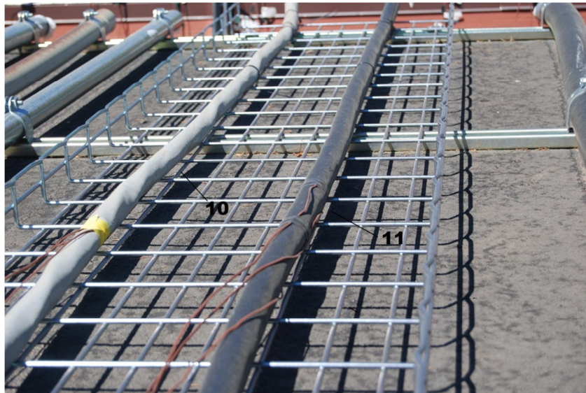
Fig. A4 – No. 1/0 SE (10), No. 1/0 TC (11), Installed in Cable Tray
